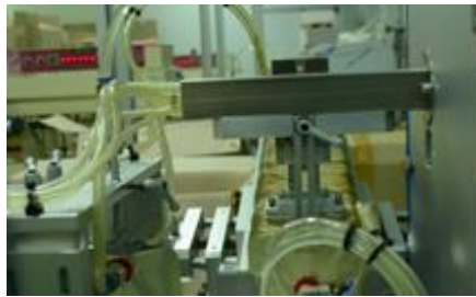
[Manufacturing and Process Facility(auto filler)]
